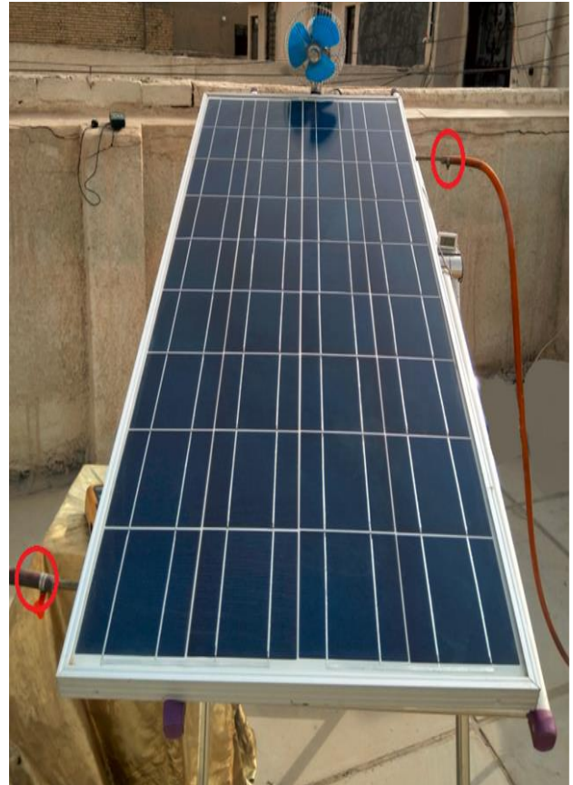
Figure 14. A visual demonstration of the installation of solar panel for Case C from front view.
