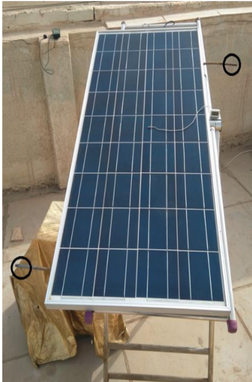
Figure 2. A visual demonstration of the installation of solar panel (Case A) from front view
